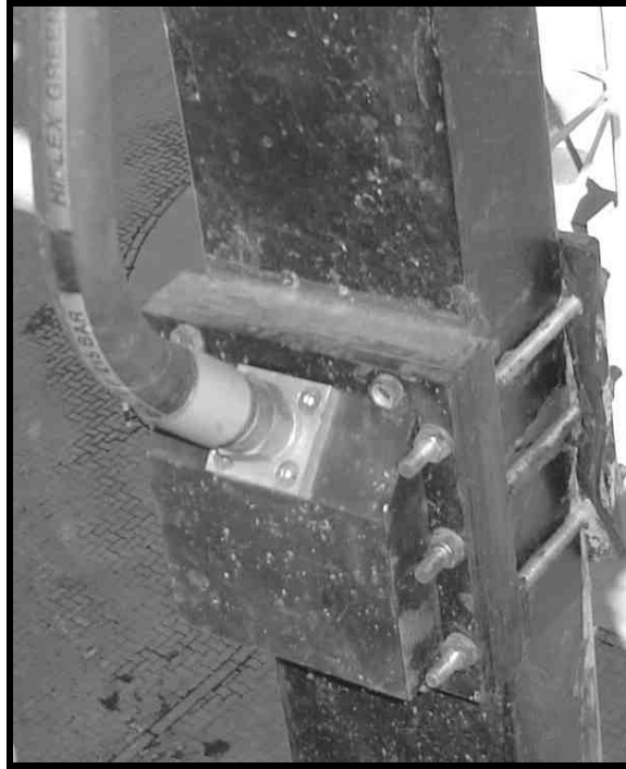
Figure 4: A Blue Cube Scanner head installed in a slurry stream
